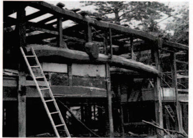
屋根を降ろして取り払うと巨大な梁が現れる With the roof and walls removed, an impressive horizontal beam is exposed to view
